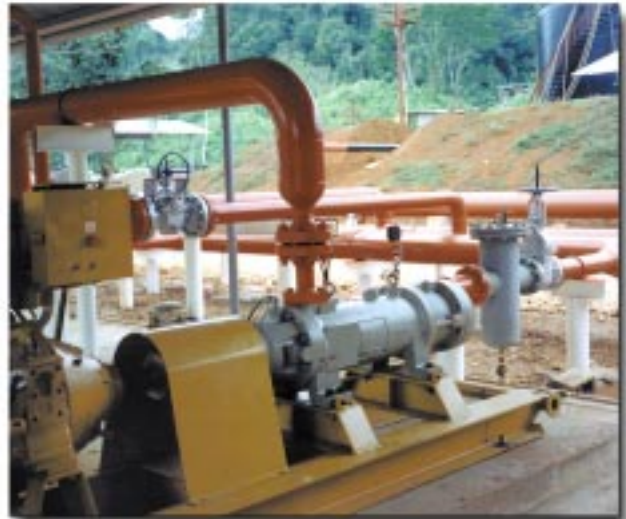
Diesel engine drive 8L-400 pumps on pipeline service in Central America delivering 14,000 B/D of 9300 SSU crude oil at 1400 PSIG
