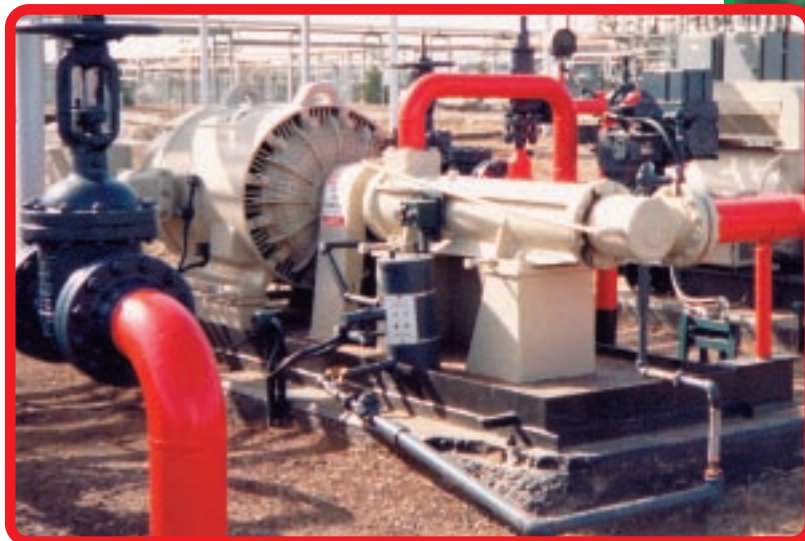
12D-400P on crude oil pipeline service in Alberta, Canada at 1440 PSIG (99 BAR)
