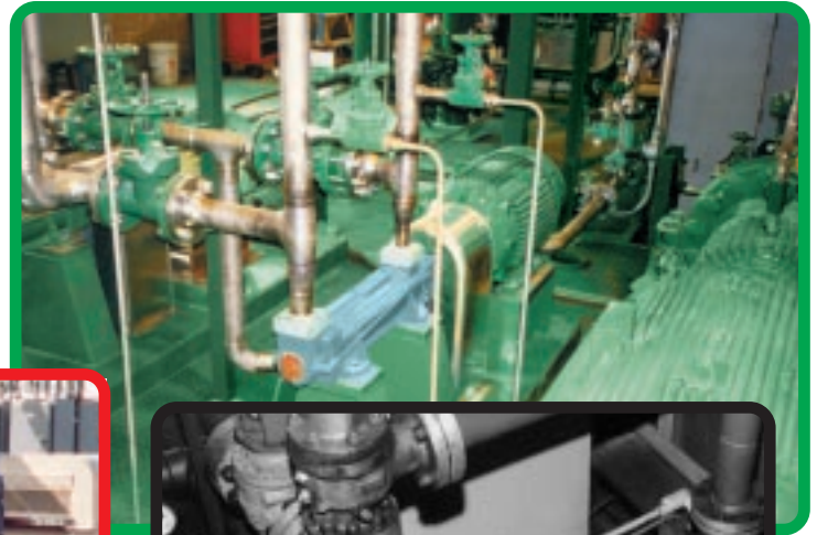
12D-137 pump on compressor gas sealing service
